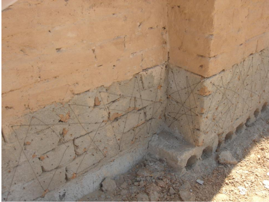
Figure 5.19: Illustrates Install mesh on the bottom of the wall to protect it from moisture (Taken by the researcher, 2011)
