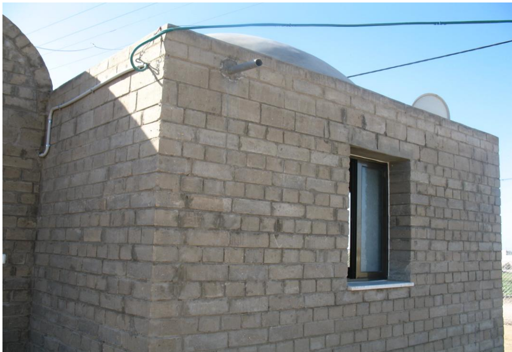
Figure 5.8: External electrical connections in the building
